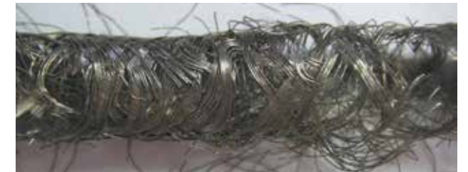
The detail inspection of the shield braid shows damage on the shield strand wires.
