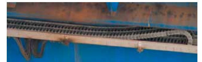
An igus® energy supply system with a length of approx. 26m in a stainless steel trough.
